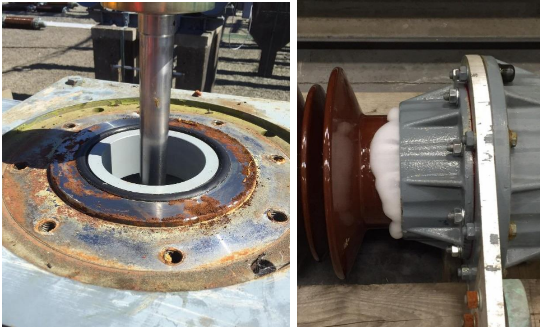
Figure 6.5: Photos of leaking FE circuit-breaker
