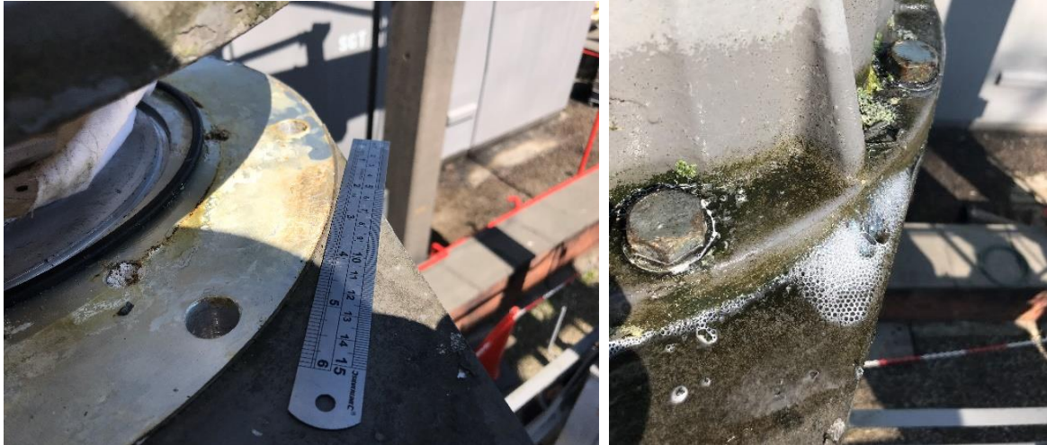
Figure 6.3: Photos of leaking SF6 circuit-breaker
