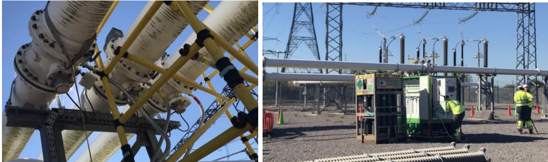
Figure 7.8: Retro-fill of SF 6 with alternative gas.
