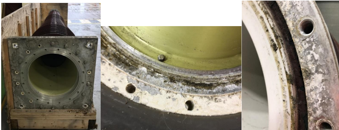
Figure 6.6: Photos of leaking [REDACTED] bushing
