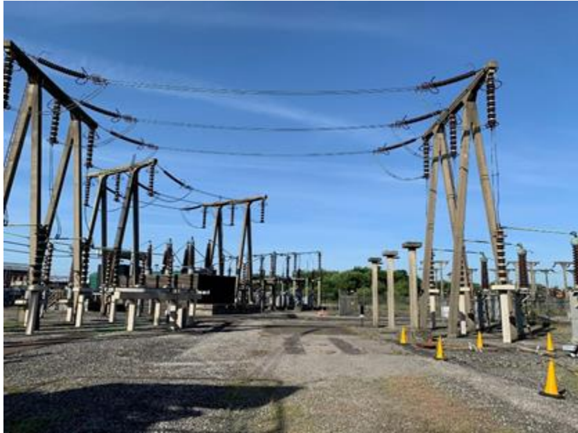
Figure 6 – Lister Drive – Birkenhead circuit overhead busbar section
