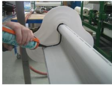
Sheds are slid down over the horizontal profile and sealed with silicone
