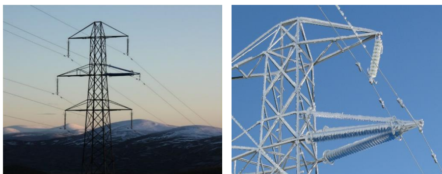
Figure 28 – Photos of Lecht installation
