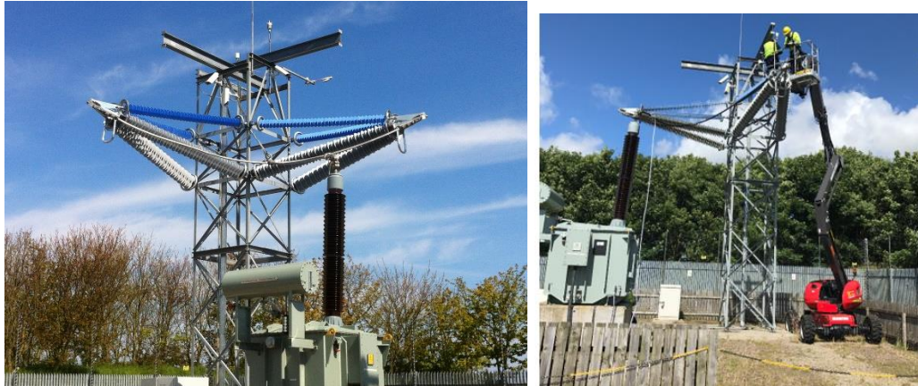
Figure 30 – Test tower with ICAs at St. Fergus.
