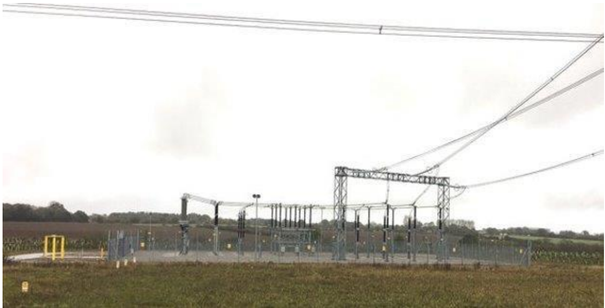
Figure 3.2 Cable Sealing End Compound with gantry
