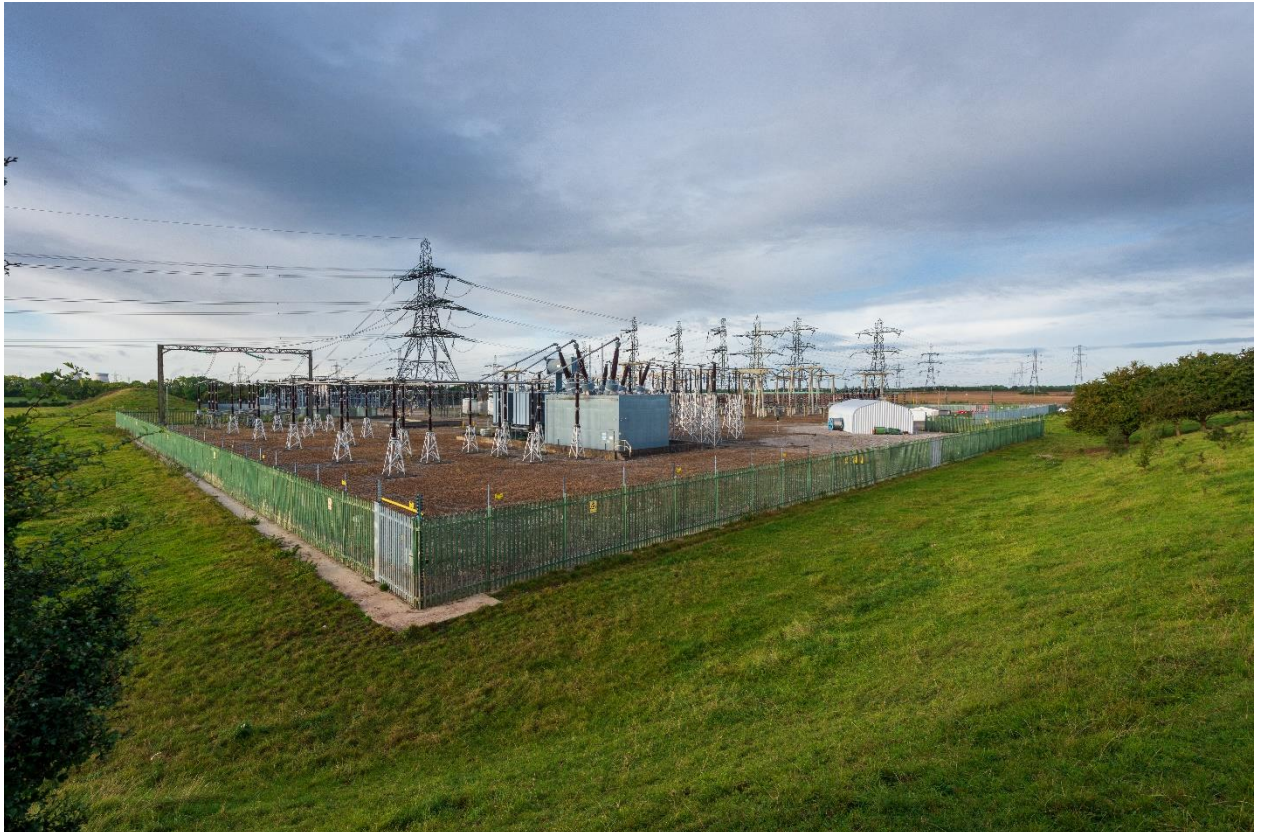
Figure 3.4 Typical Substation (existing Monk Fryston Substation)
