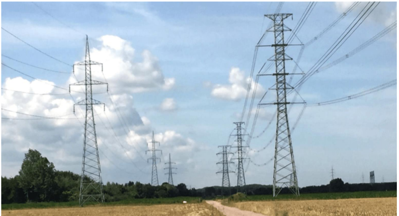
Figure 2.9 - Pre-existing 150 kV line (left) and new 380 kV compact line with ICAs (right) [13]
