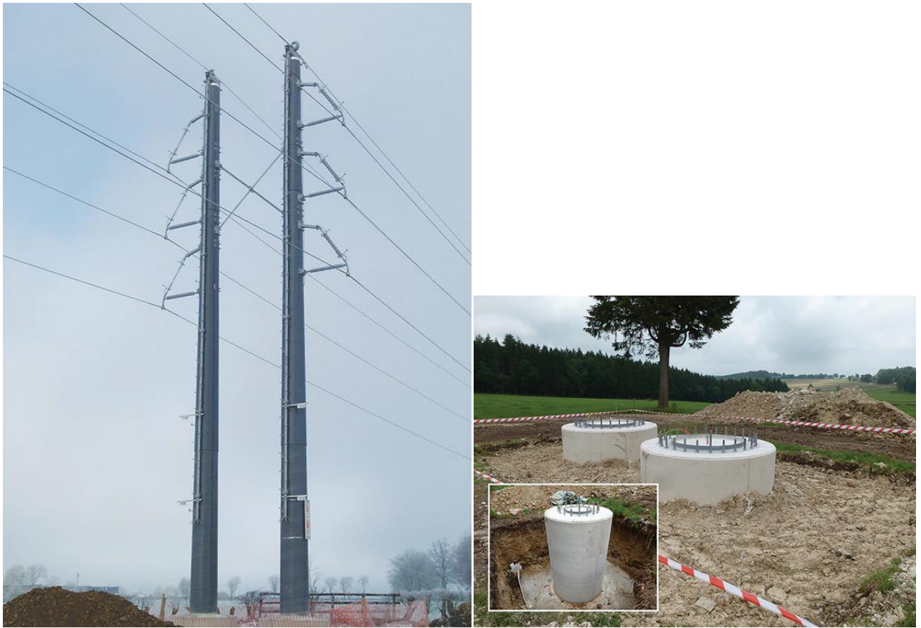
Figure 2.8 - Composite gantry poles with ICAs (left) and tower foundations (right) [11]
