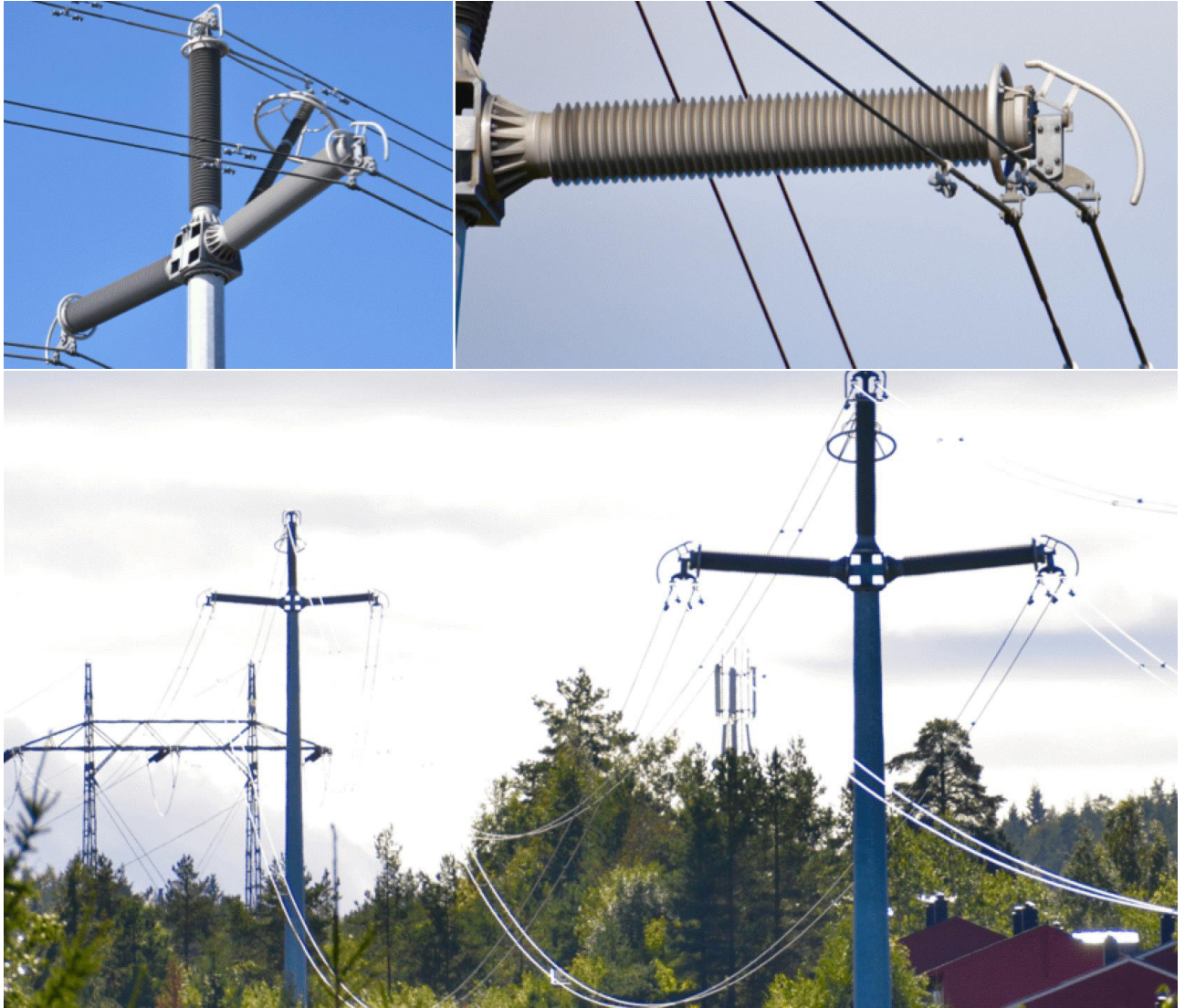
Figure 2.17 - 400 kV compact OHL test span at STRI using foam-filled hollow core post insulators
