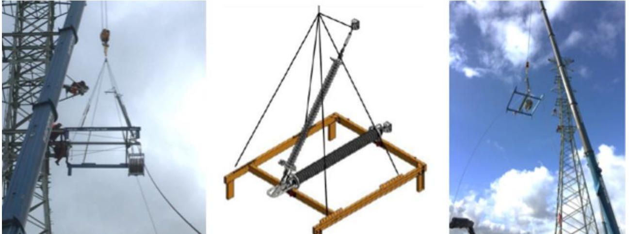
Figure 2.10 – ICA installation using flexible mounting platform [13]
