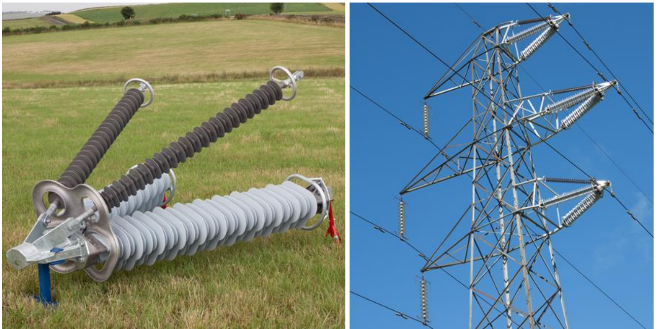
Figure 6.5 - 132 kV ICA (left) and three ICA installed on a live OHL (right) [4]
