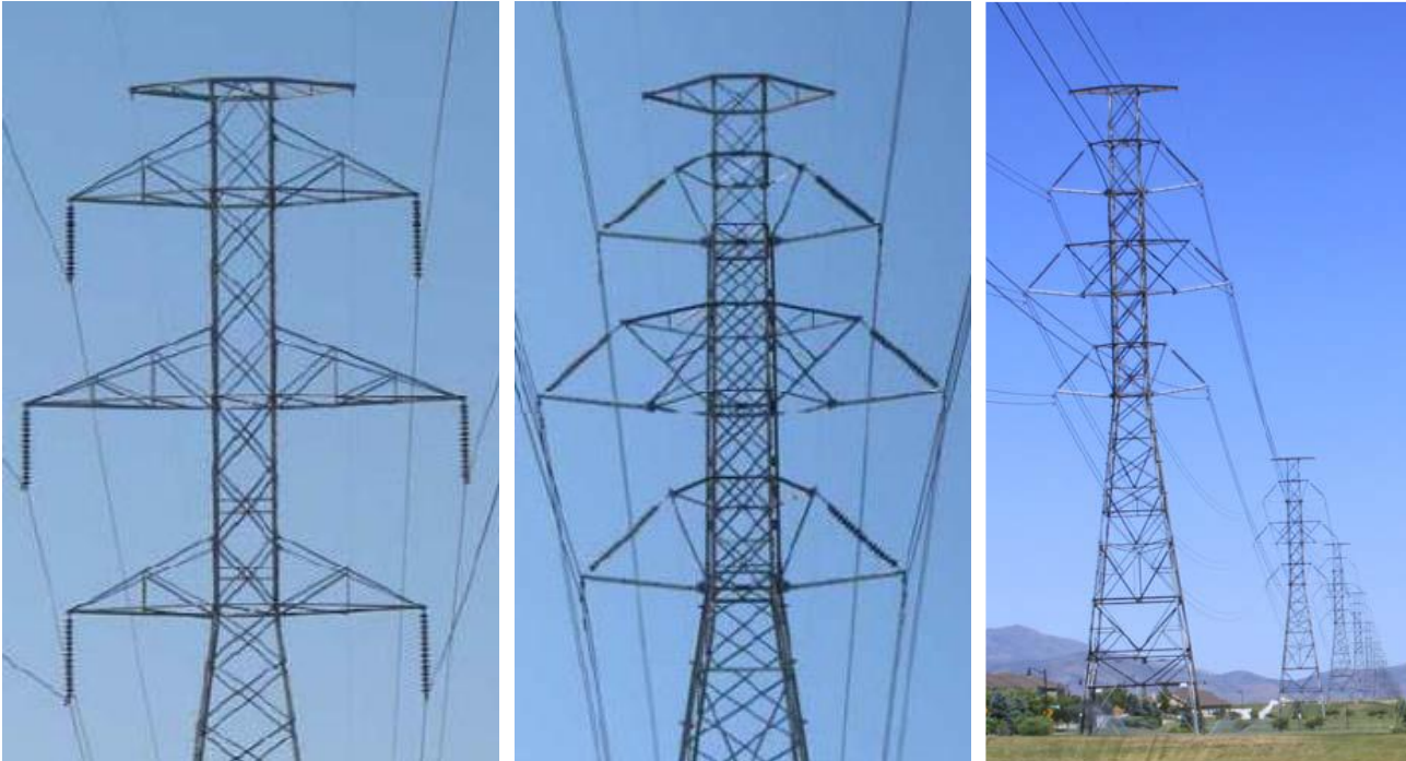
Figure 2.4 – Existing 230 kV OHL (left), uprated 345 kV OHL with ICAs (right)
