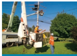
Electricity Distribution & Generation 66-73
