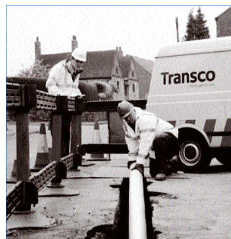
Above UK gas mains replacement work at Hatham, Leicestershire, which is part of our ongoing national mains replacement programme to make the network safer.
