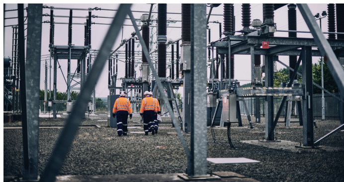
A National Grid AIS substation - for illustrative purposes only.
