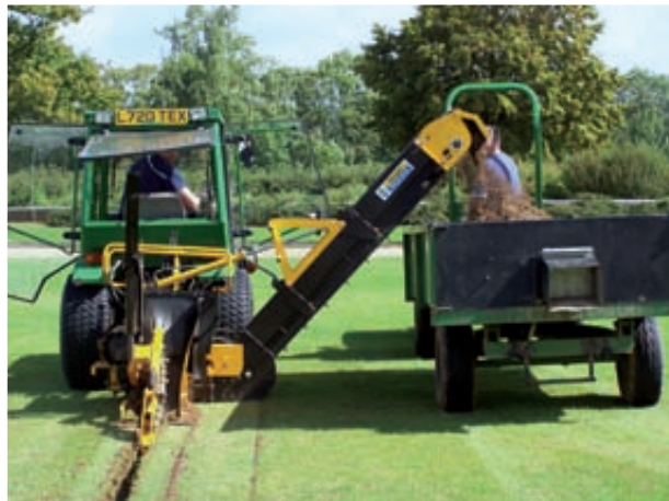
DIGGING DEEP: The AFT 100 Trencher (above) installs field drainage systems in one pass, but the excavating teeth can penetrate to a depth of 1.6 metres – bringing them into the potential zone of pipelines (left) Compact trenchers are used for sports fields and golf courses where it is vital to minimise disruption
