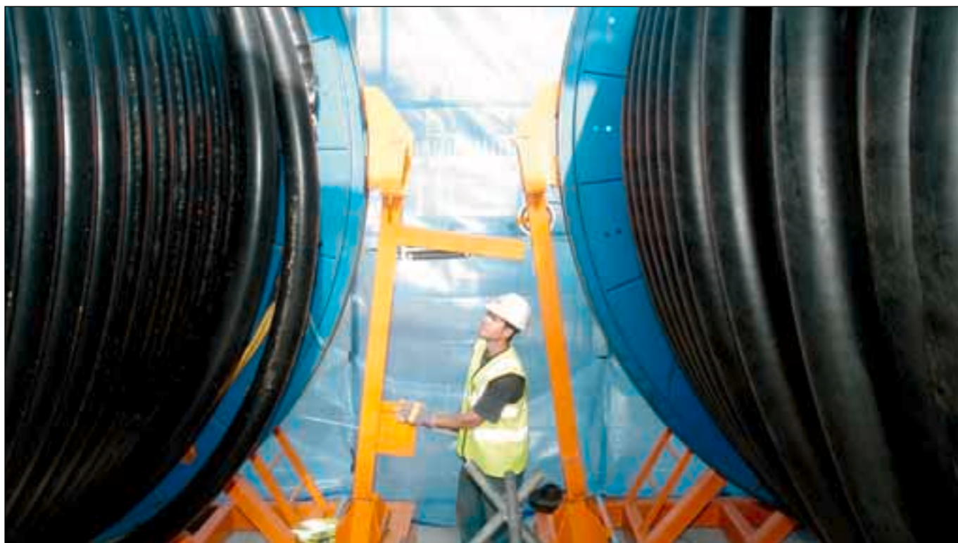
A worker is dwarfed by the cable, which arrived in 950-metre lengths on 63 drums, each weighing 44.5 tonnes
