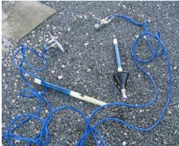
Figure 6.2A - Temporary Earth Bond and Pole
