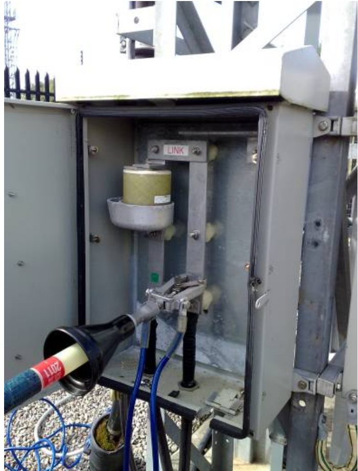
Figure 6.1C - Temporary Earth Bond
