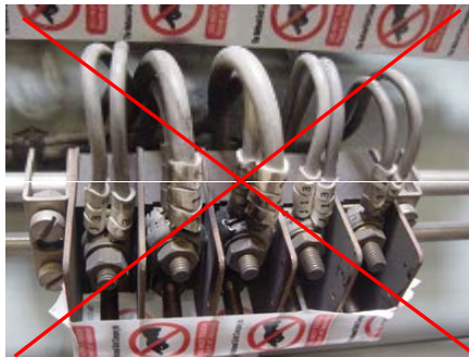
Figure A1 – Example of Incorrect Screening Material and Screening
