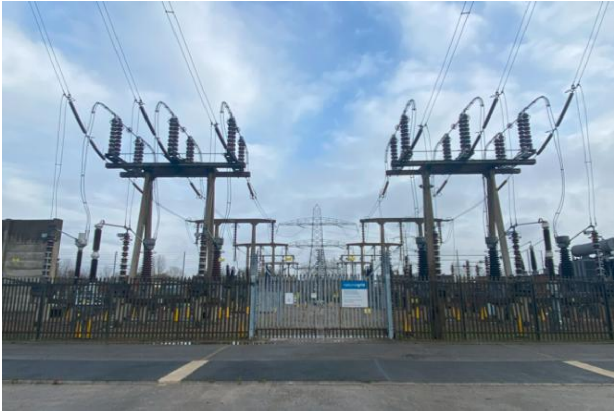
Above: An image of National Grid's Templeborough substation in Tinsley, Sheffield.
