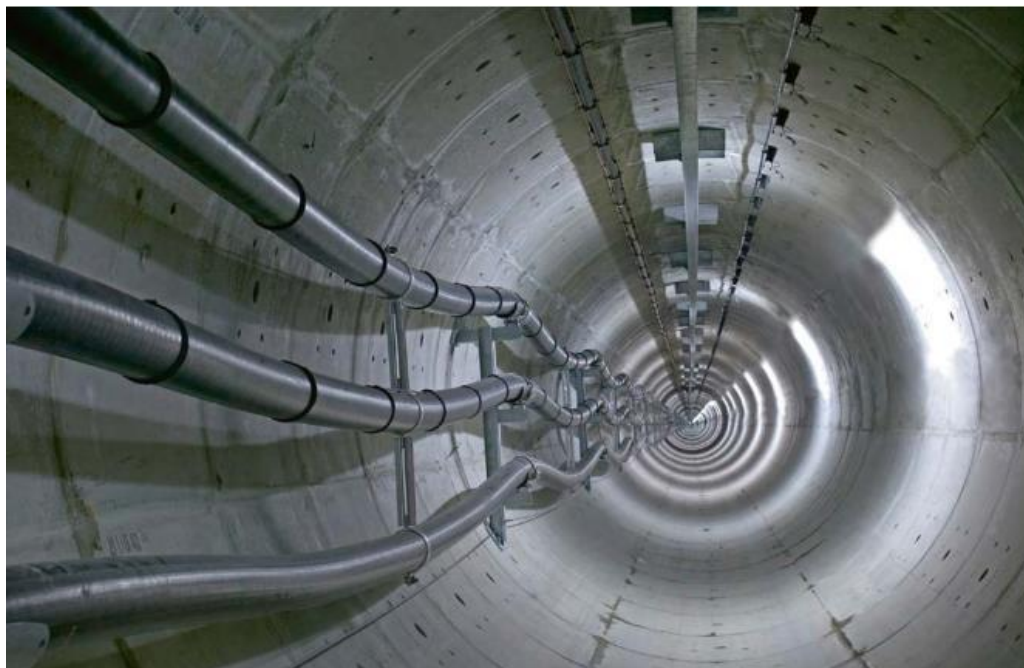
Figure 3-1: Example of XLPE Cables installed in a deep bored tunnel
