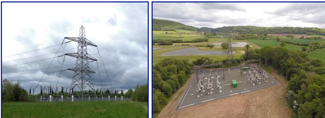
Figure 2.4 – Example 400kV Sealing End Compounds
