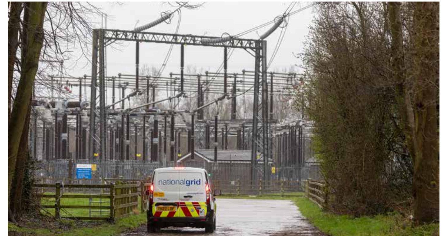
Example of a 400 kV substation for illustrative purposes only.
