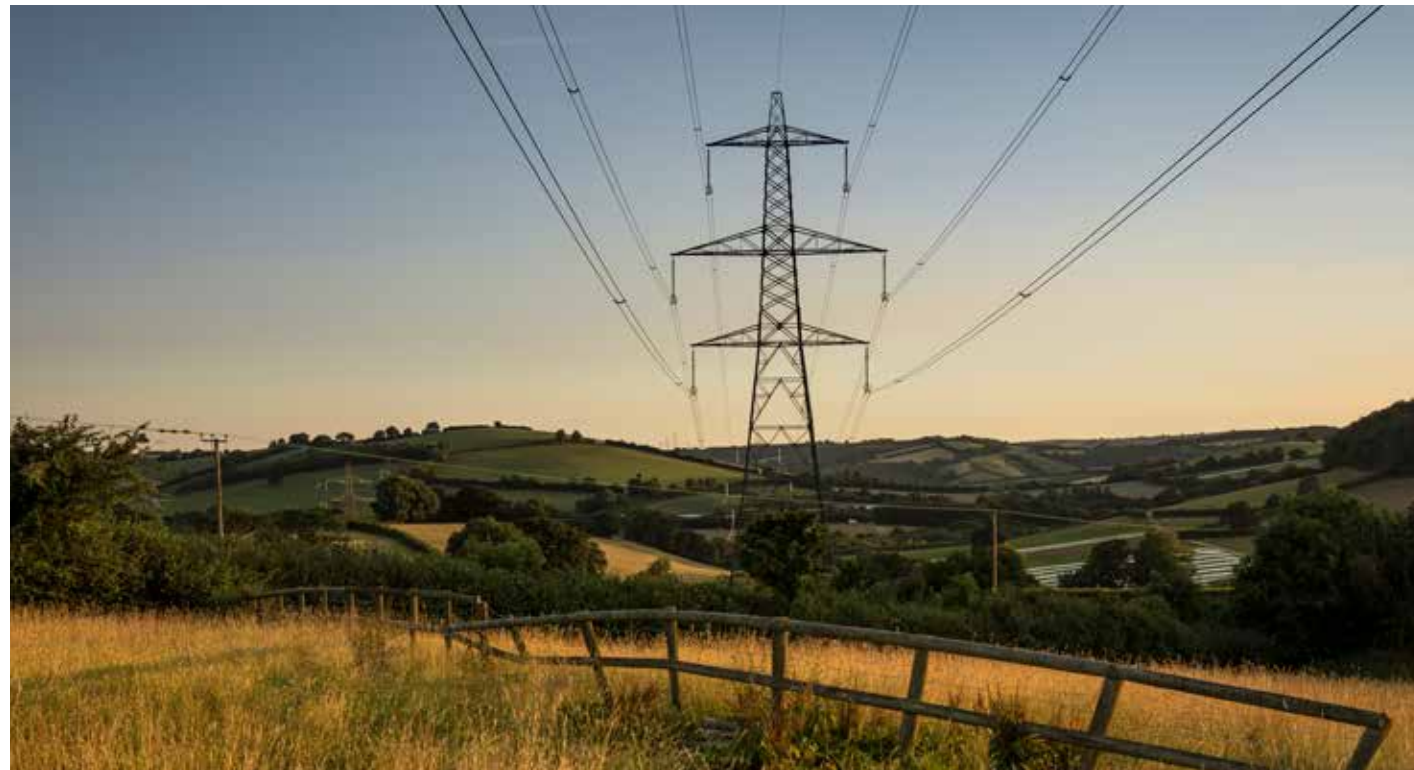
Example of 400 kV overhead line and pylon for illustrative purposes only.
