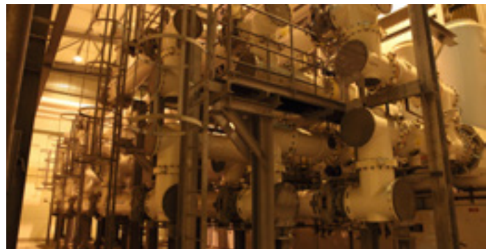
A National Grid GIS substation - for illustrative purposes only.
