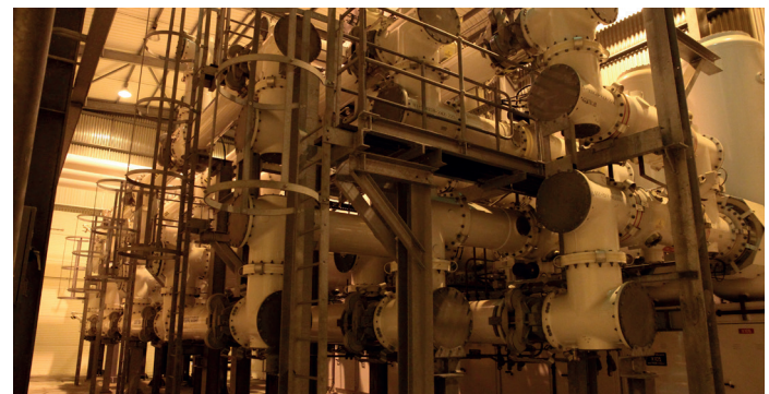
A National Grid GIS substation - for illustrative purposes only.
