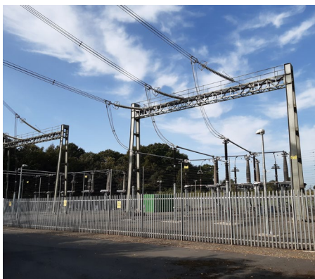
Cable sealing end compound
