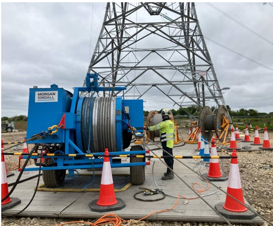
Fig10. Typical Work Setup at conductor pulling locations shown in hatched purple in Fig9.
