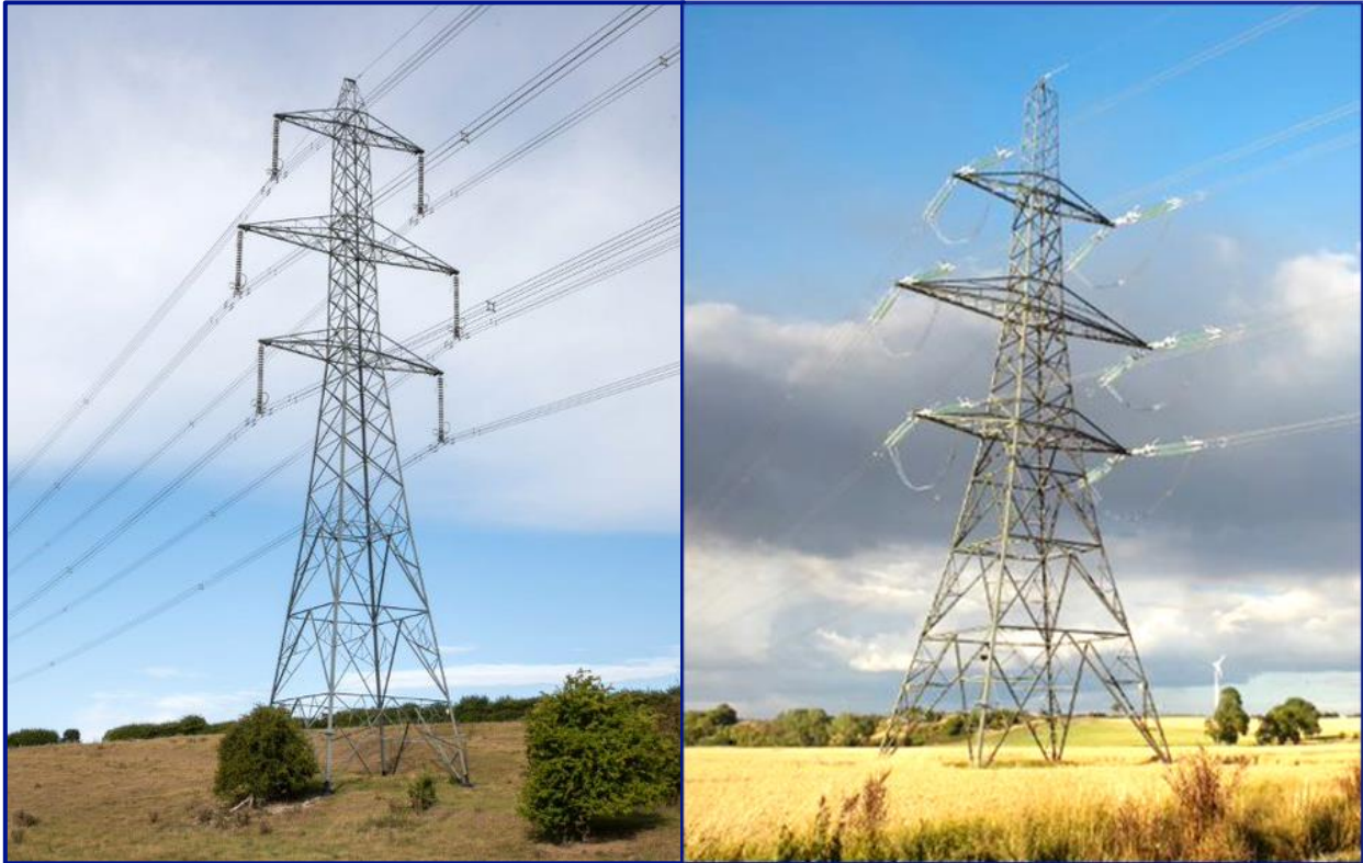
Figure 2-2 – Suspension Pylon (Left) and Angle Pylon (Right)
