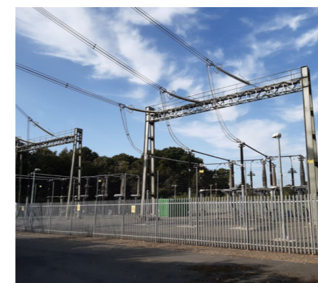
Cable sealing end compound
