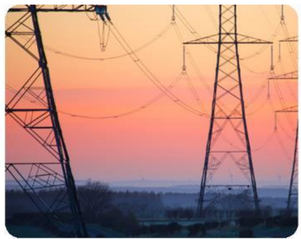
National Grid Pylons and Overhead Lines
