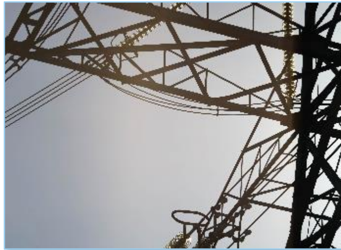
Electricity Distribution (ED) (previously WPD)
