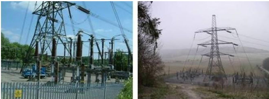
Figure C.5: Cable Sealing End Compounds
