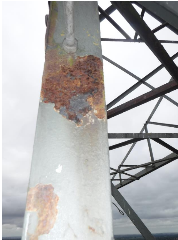
Figure 6.1: Typical grade 5 rust patch on Leg Bars (ZL061 – photo DSCF9174)
