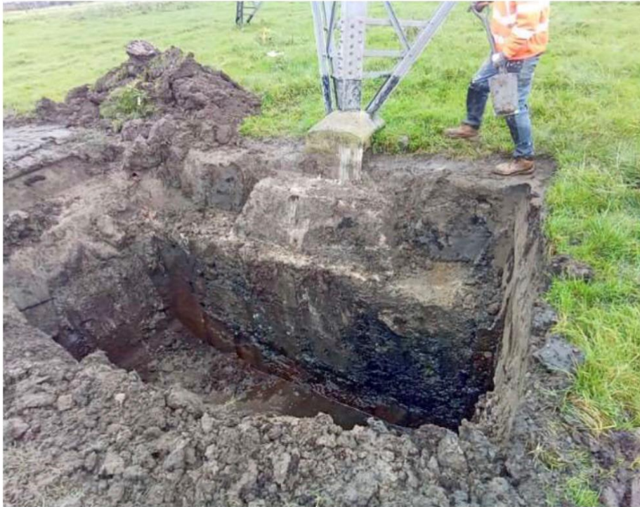
Figure 6.8: Extract from EJR for 4ZE015 showing honey-combed concrete
