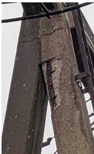
Image 2: Reinforced Concrete Support Structure Defect
