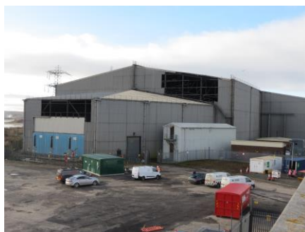
Image 3: Missing cladding at Blyth Substation
