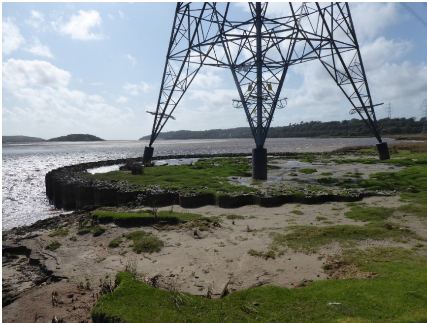
Plate 15.7: Pylon 4ZC030R – scouring along the southern margin of the cofferdam
