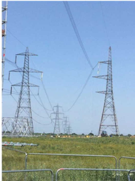
Image 2: Example of a 132kV Cable Sealing Platform Pylon and Downloads*
