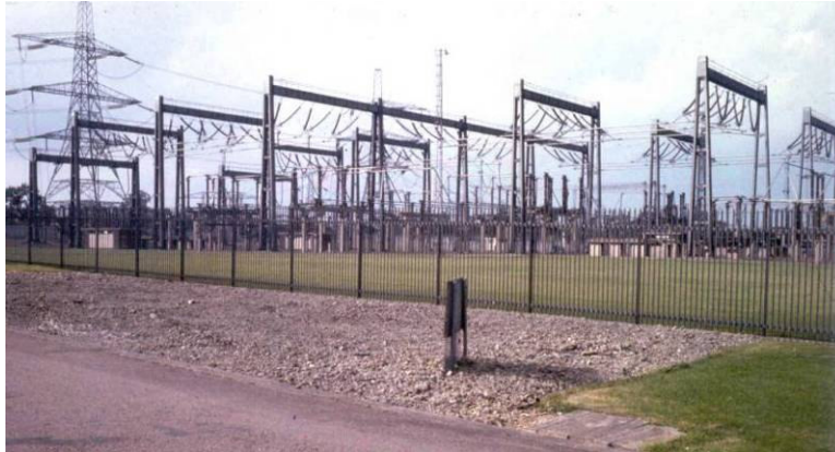
Figure 4.1.4 – 400 kV Air Insulated Substation
