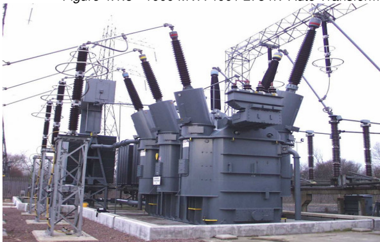
Figure 4.1.5 - 1000 MVA 400 / 275 kV Auto Transformer
