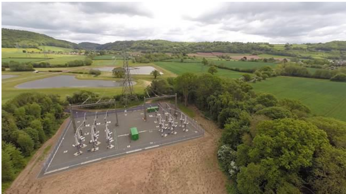
Figure 3.5 – 400kV Cable Sealing End Platform
