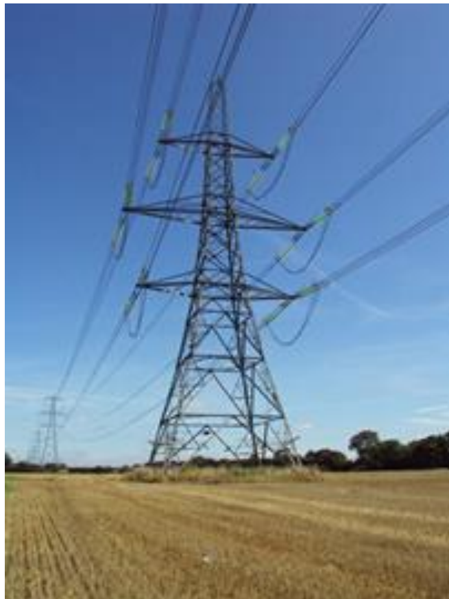
Figure 3.2 – 400kV Steel Lattice Angle Pylon
