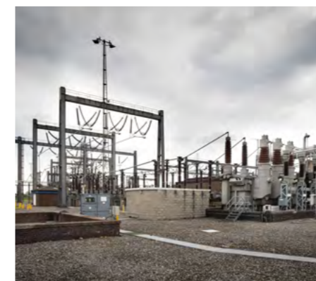
Cable sealing end compound
