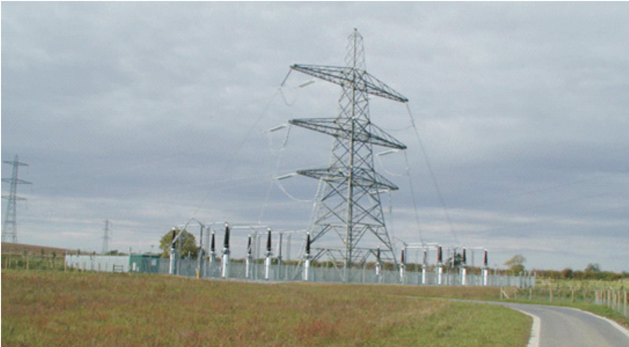
Photograph indicative only and final design of cable sealing end compounds may be different
