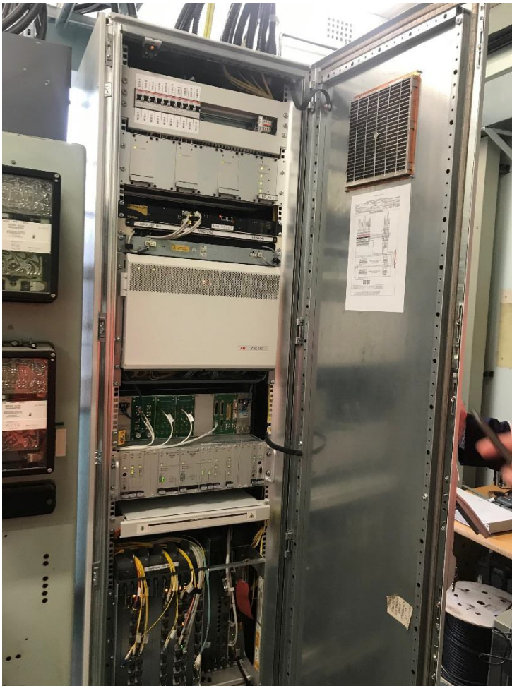
Figure: Photo of a typical OpTel network equipment cabinet at an NG substation
