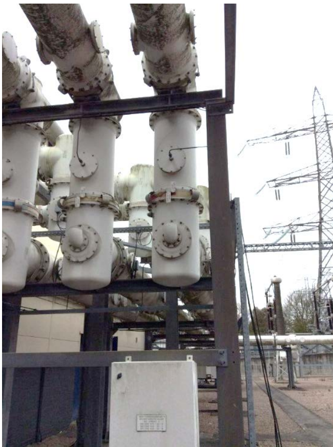
Figure 11 – 19 year old YG3 design GIS at Northfleet East showing evidence of corrosion
