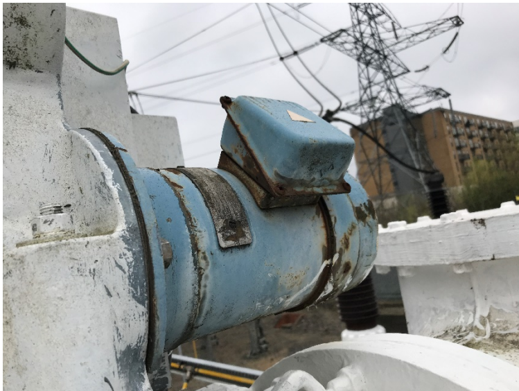
Figure 12 – 31 year old 275kV SP1 at Wimbledon showing evidence of corrosion
