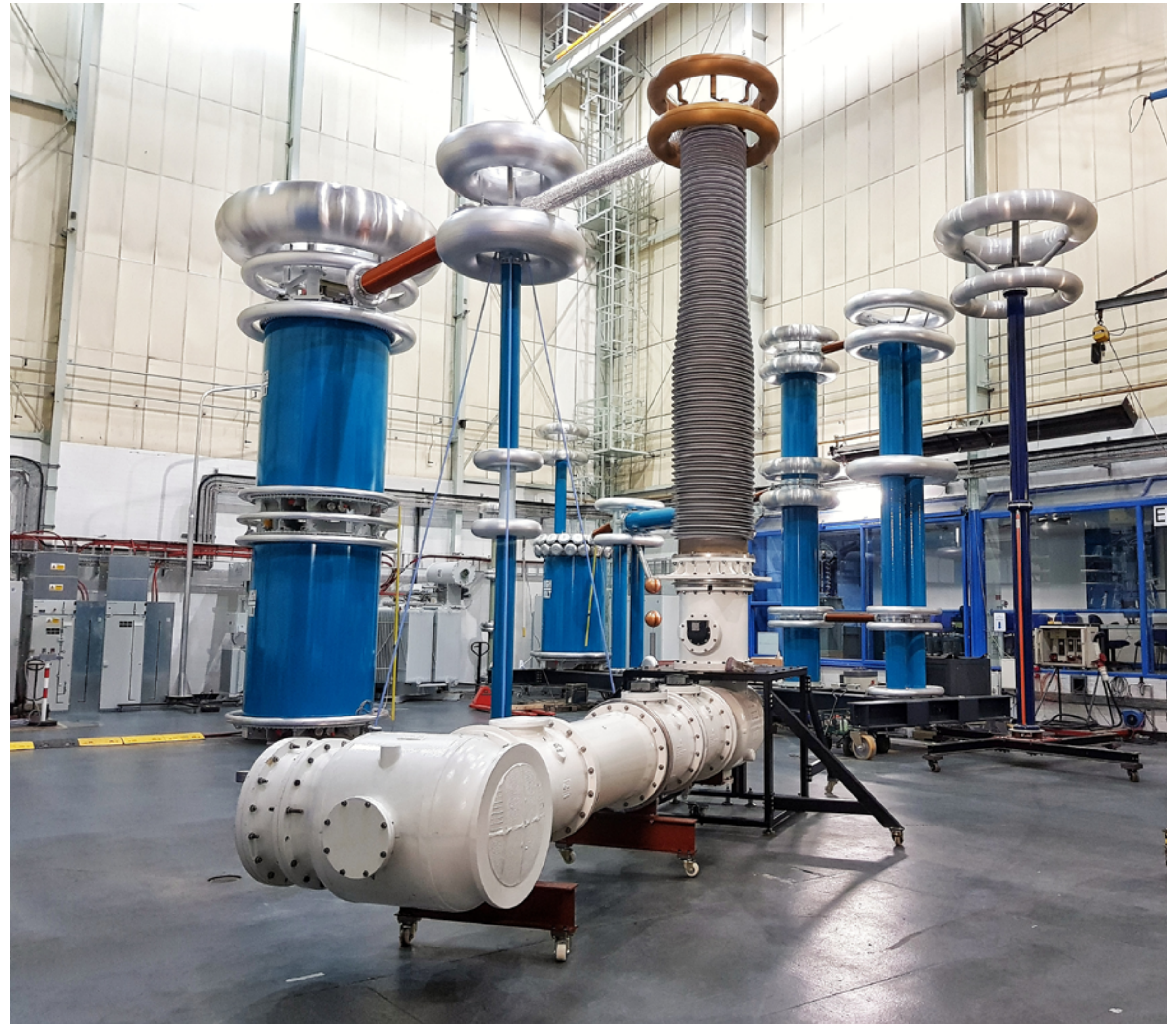
The gas-insulated bus bar demonstrator that NGET is using to conduct its research into SF 6 alternatives
