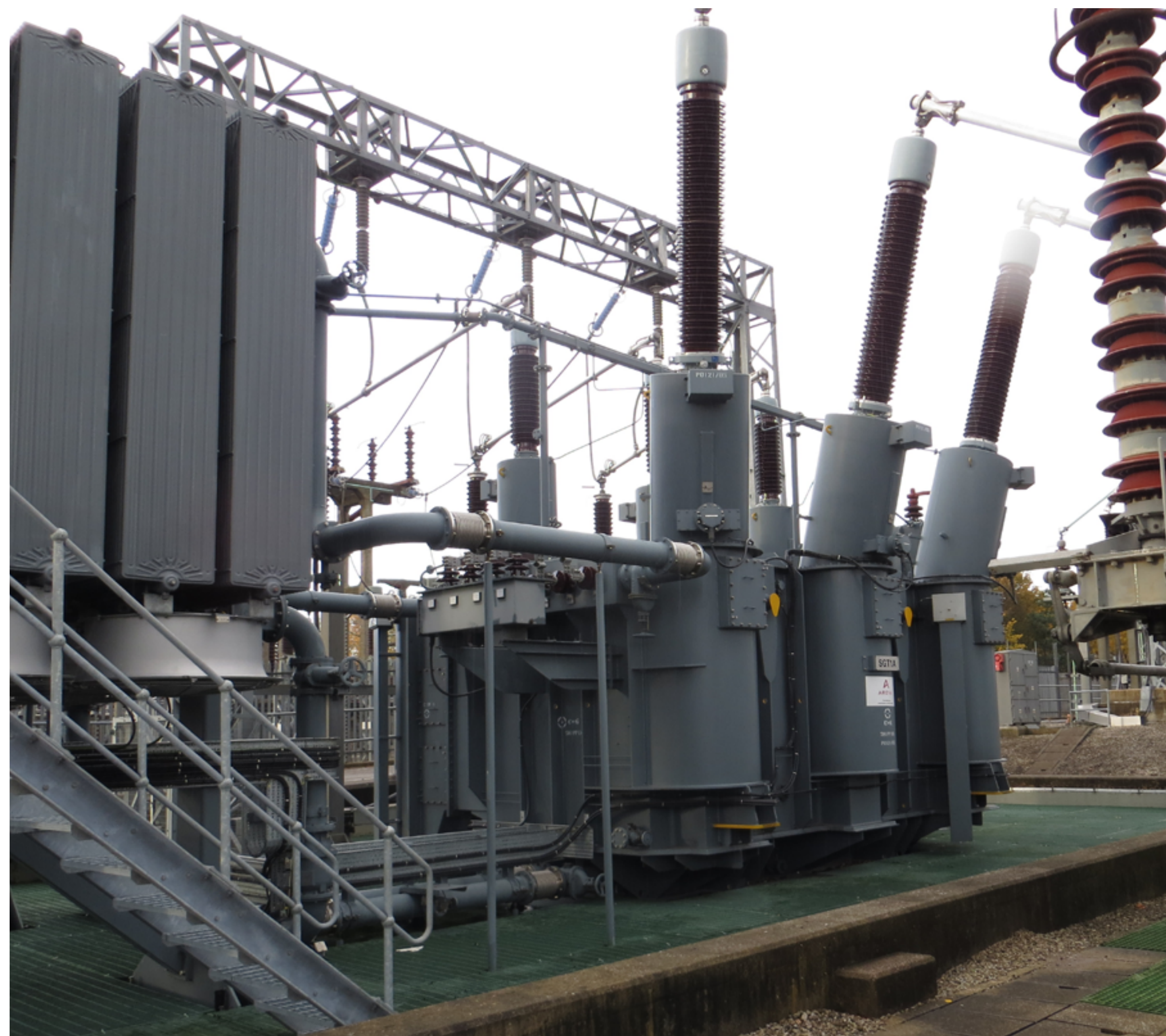
The ConCEPT project examines the ratings capability of our transformers
