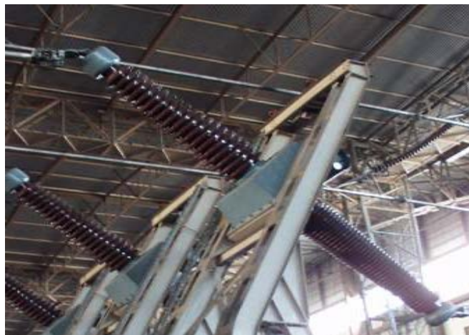
Figure 1 – Photograph of a 400kV through wall bushing
