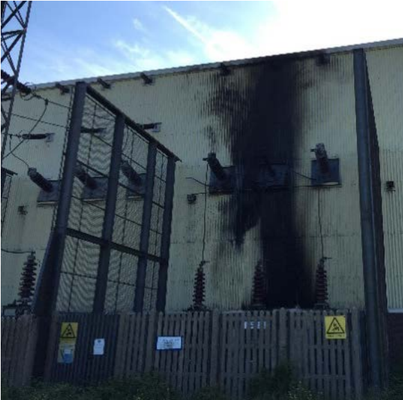
Figure 2a - External burning & carbonisation of substation wall
