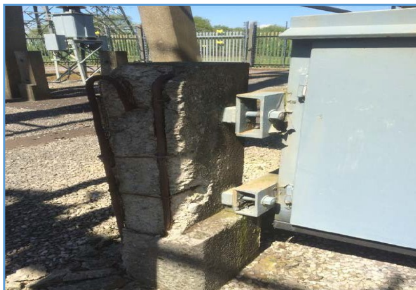
Figure A3: Corrosion of concrete structure.
