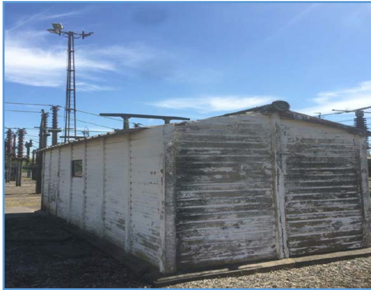
Figure A2: Deteriorating buildings
