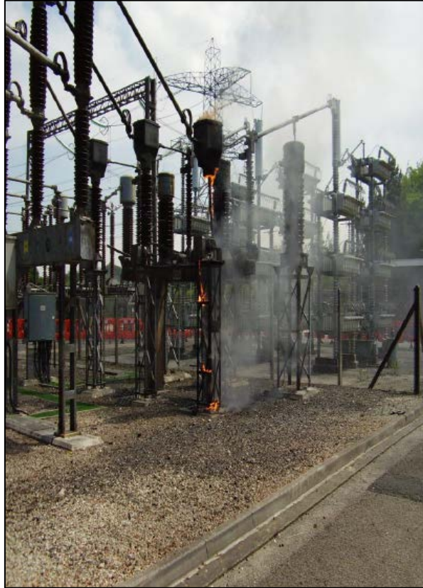
Figure 3 – Catastrophic failure of FMJL CT. The porcelain insulator exploded firing shrapnel across the site.
