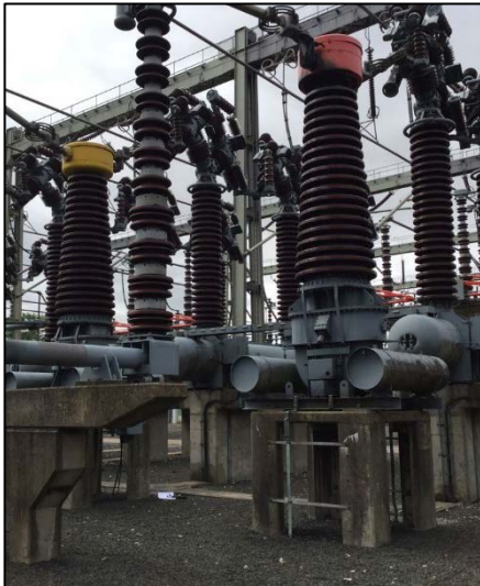
Figure 1 - 400KV Hairpin CT at Cottam 400kV Substation
