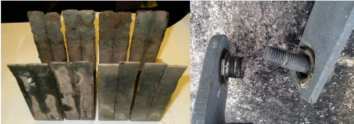
Figure 2: Example of disconnecter contact corrosion and a broken drive linkage
