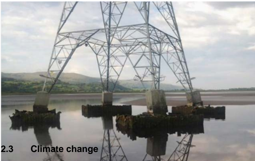
Figure 1: Visual example of the impact of erosion on towers
