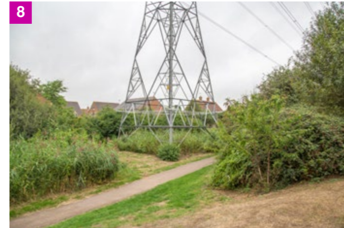
8 Planting around the base of the pylon limits views of the structure and provides a high degree of sensory richness. Importantly easy access is possible for maintenance of the pylon and overhead wires.
