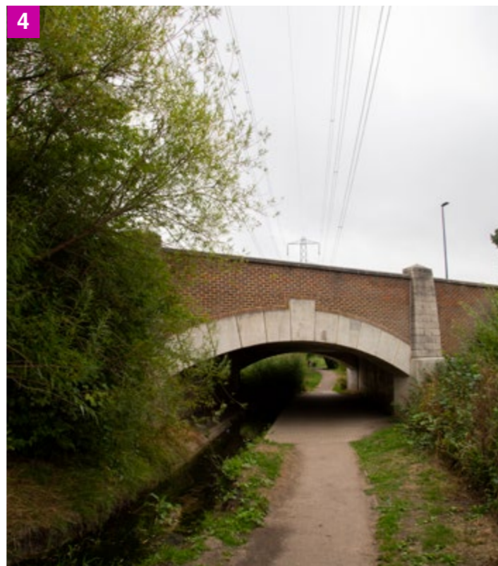
4 While their design provides relatively little sensory richness, the road bridges - providing essential vehicular connectivity across the transmission line - create thresholds and provide screening of the pylons.
