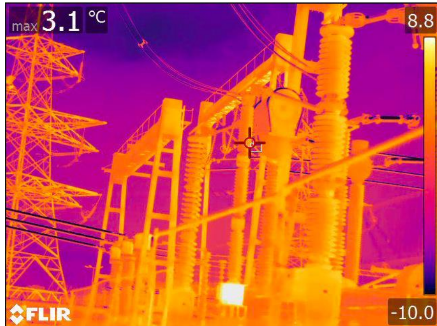
Figure 9. Condition Monitoring of substation assets via non-intrusive thermal imaging
