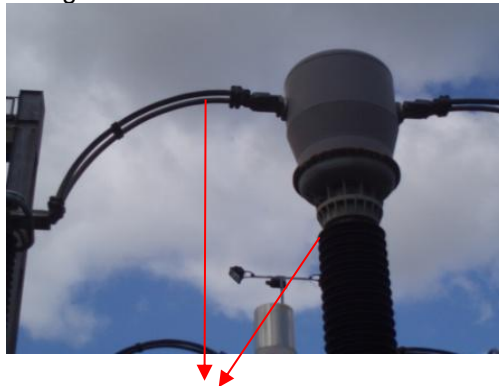
Figure 7.2A – Example of proximity of lower level equipment - Safety Distance to be maintained when applying portable Earthing Device(s) will be from the bottom of the CT housing not the conductor as indicated by the red arrows.
