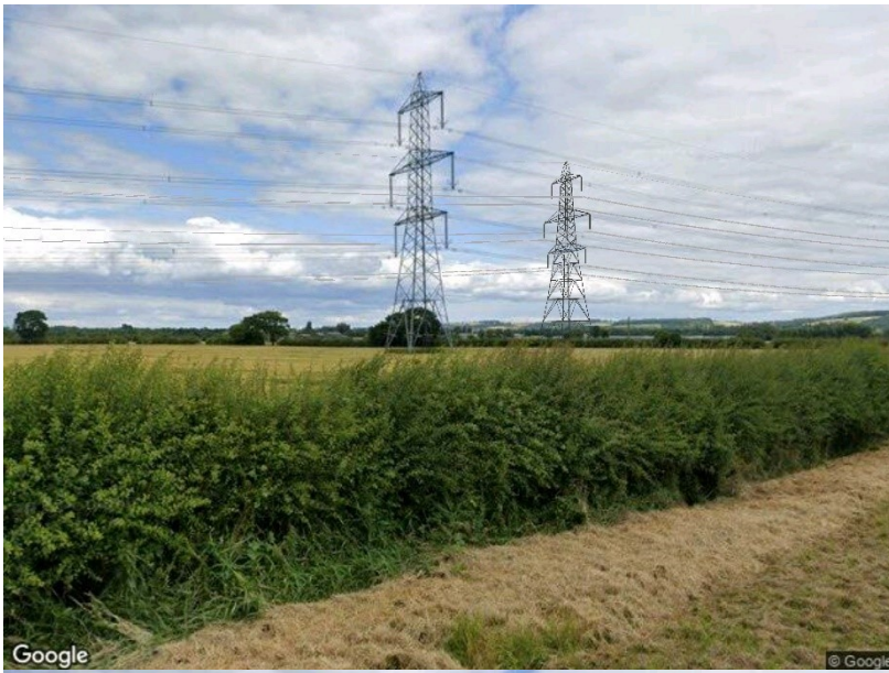
Illustrative wireline image of an overhead line constructed using the standard lattice pylon
