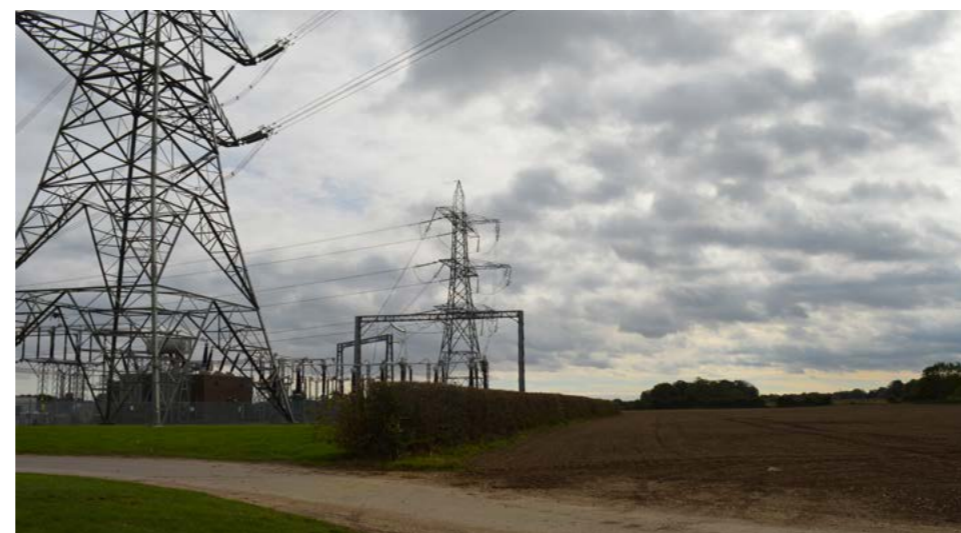
Pylons converge on Creyke Beck Substation which is located on the southern edge of this LCT
