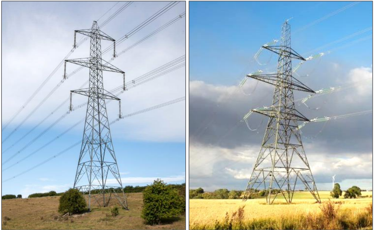
Image 4.3 – Suspension pylon (left) and tension pylon (right)
