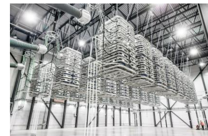
Converter Valve Hall
