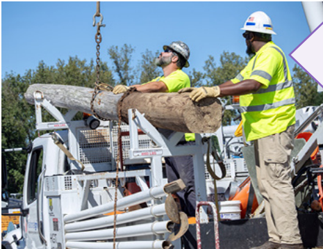
US field force working on the local electricity system, delivering the investment required across the distribution network.
